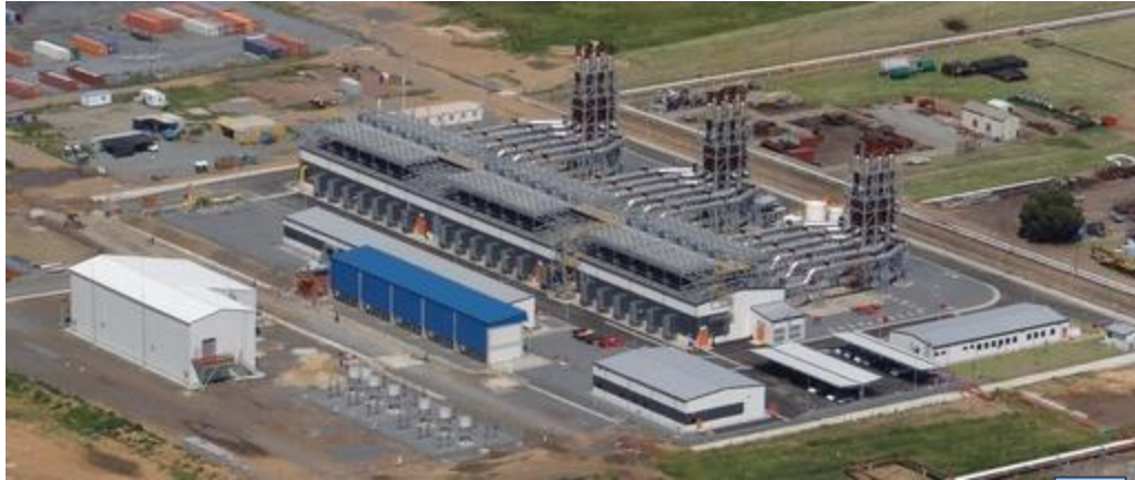
Sasolburg Gas Engine Power Plant 18 Wärtsilä 34 SG engines (140 MW) Largest plant of its kind in Africa Highly efficient and environmentally friendly facility Inaugurated July 2013
